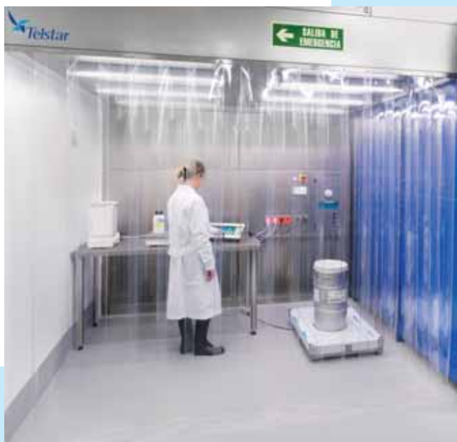
Compact SS 304 recirculation downflow booth installed inside the warehouse
